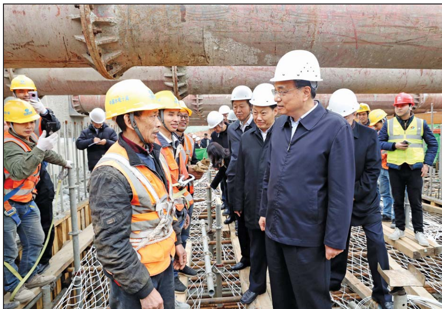
Premier Li Keqiang, visiting a construction site on Monday in Chengdu, Sichuan province, talks with migrant workers after climbing up a scaffold. He asked them about their monthly earnings and the length of their workday. He also asked whether their wages are paid on time and in full. YAO DAWEI / XINHUA
